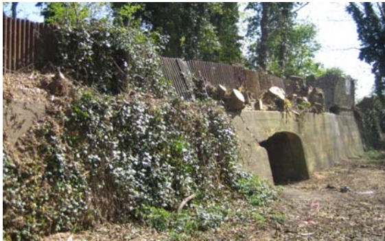
Section of raised embankment which carried tramway into Halling Manor cement works
