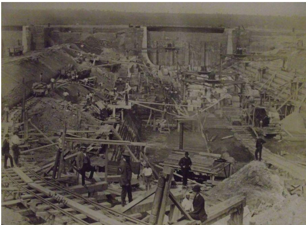
Building Dock no. 8; note the caisson is already in place as part of the basin.
